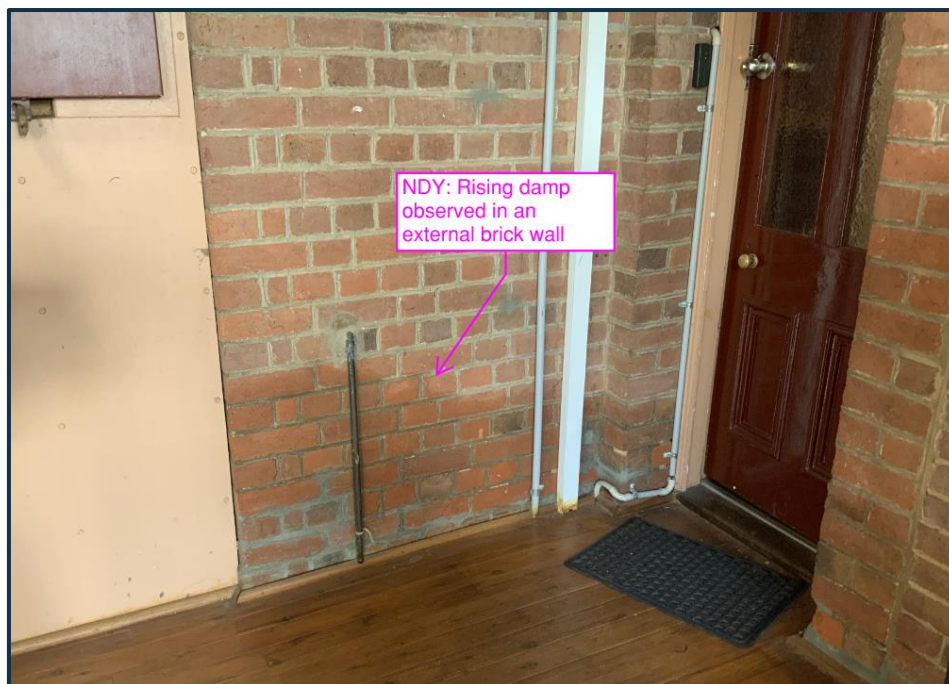
FIGURE 7 - RISING DAMP OBSERVED IN AN EXTERNAL BRICK WALL
