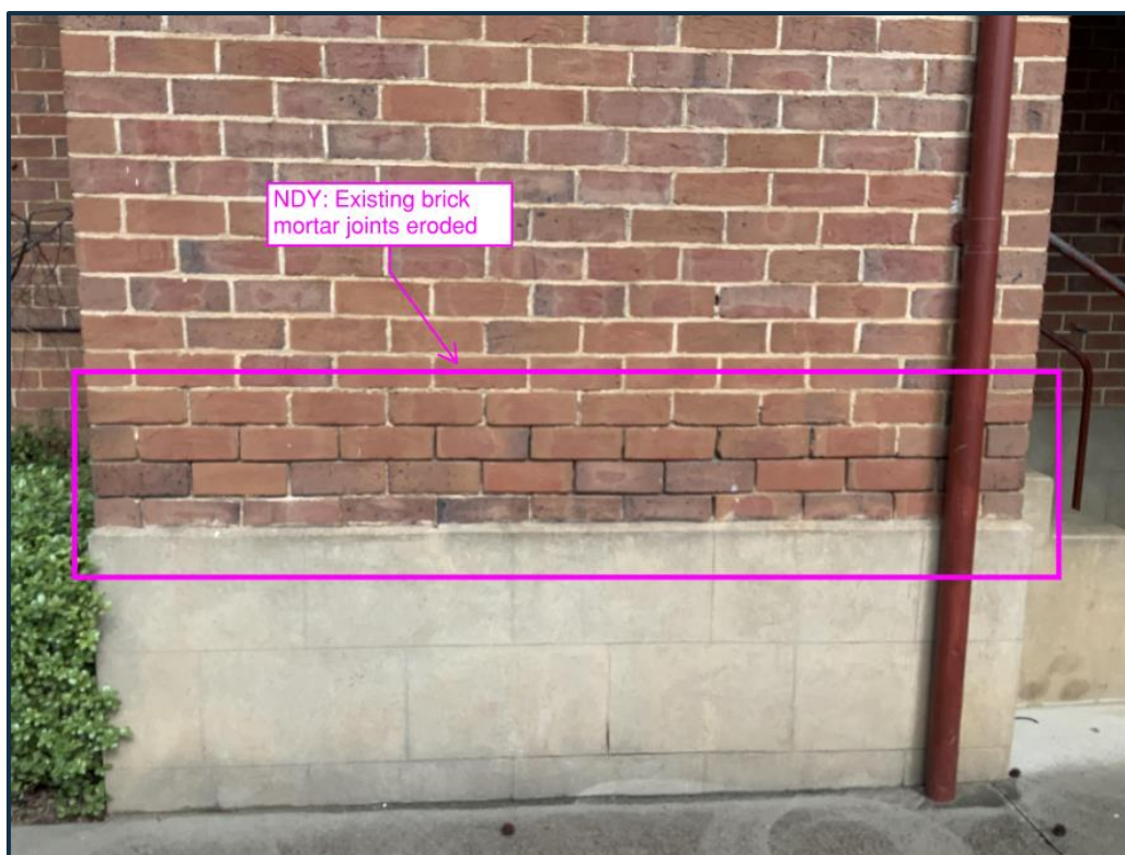
FIGURE 8 - LOCALLY ERODED BRICK MORTAR JOINTS IN AN EXTERNAL BRICK WALL
