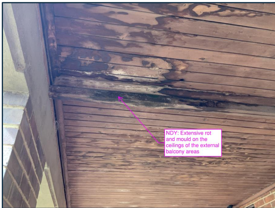
FIGURE 10 - EVIDENCE OF ROT AND MOULD ON BOTH BALCONY CEILINGS
