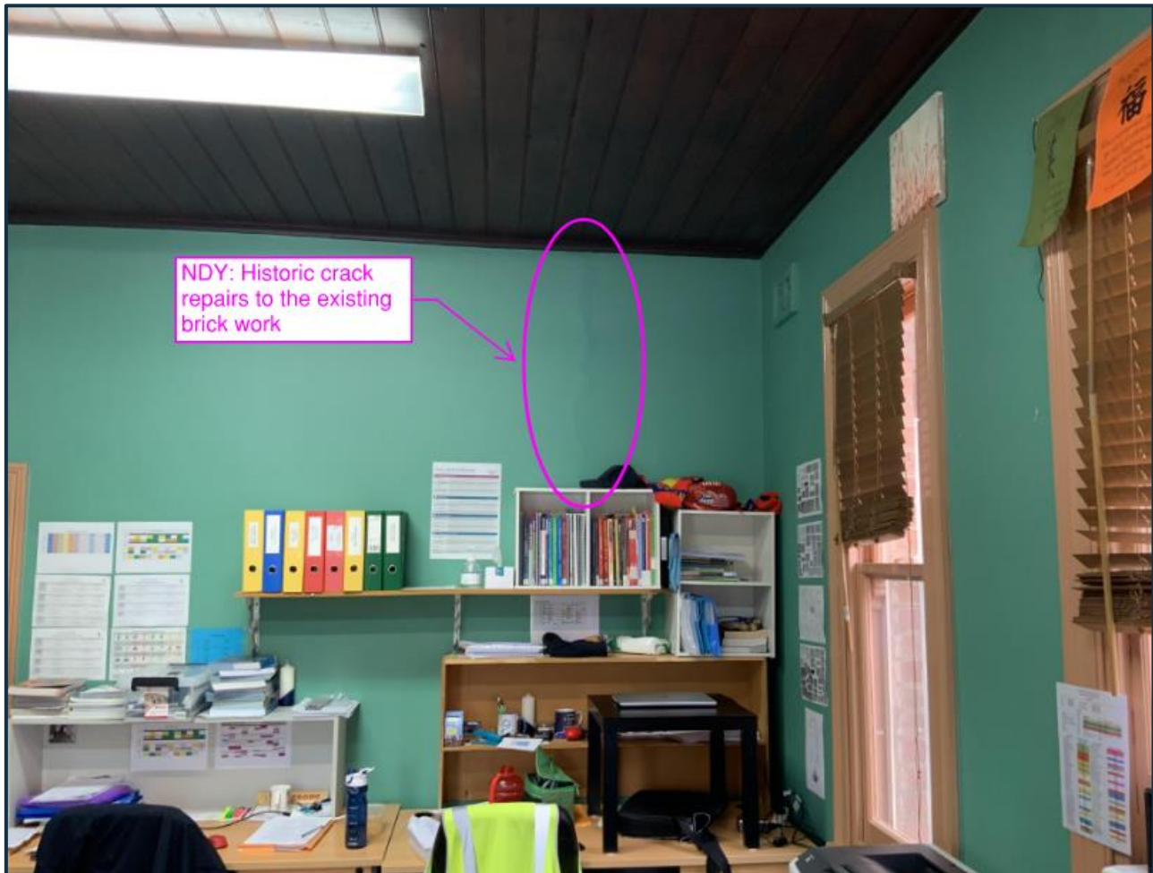
FIGURE 4 - HISTORIC REPAIRS OF CRACKING IN THE EXISTING BRICK WALLS
