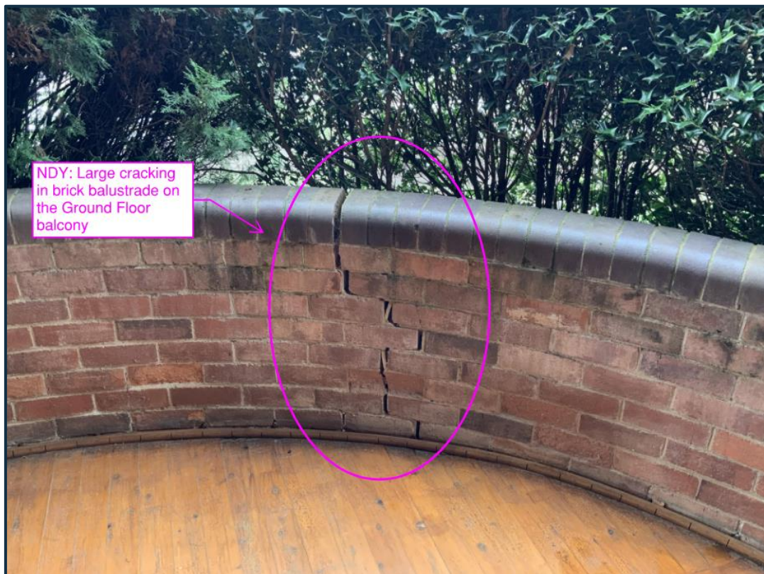
FIGURE 6 - LARGE VERTICAL CRACKING IN THE EXISTING GROUND FLOOR BRICK BALUSTRADE
