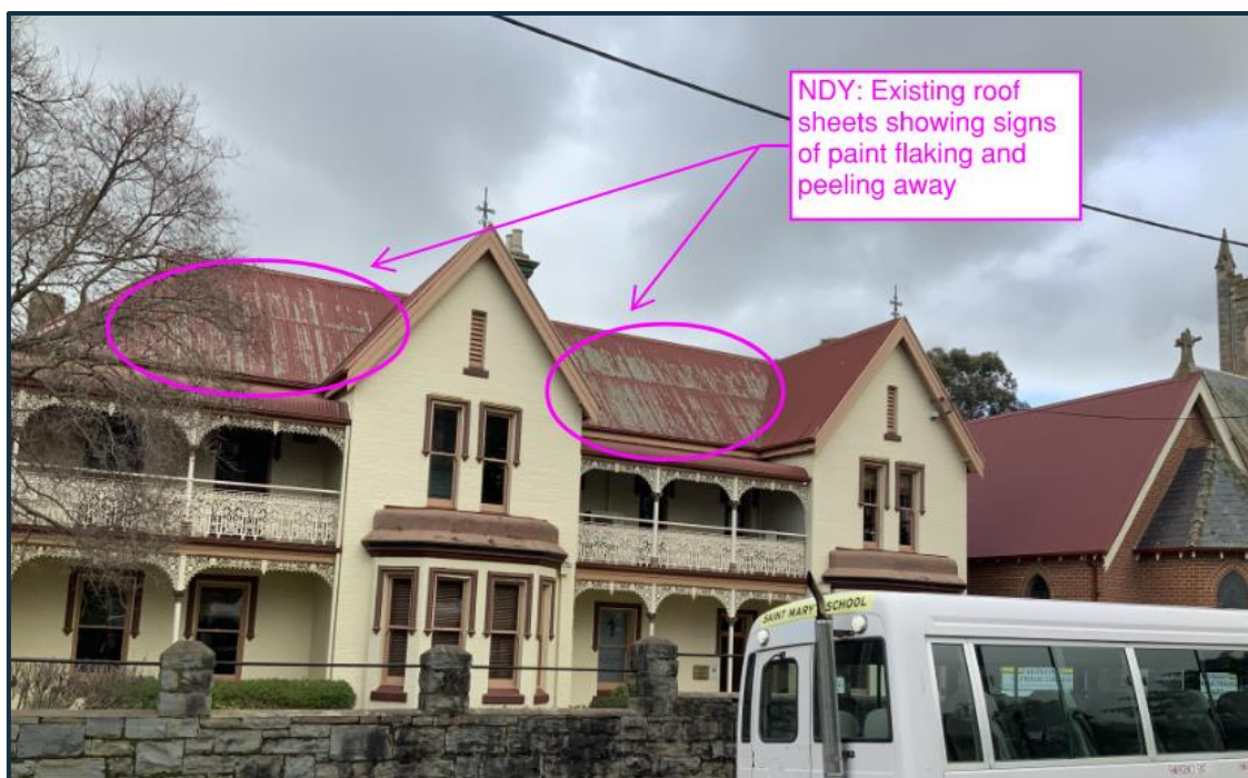
FIGURE 11 - SITE PHOTO OF THE CONDITION OF THE EXISTING ROOF SHEETS
