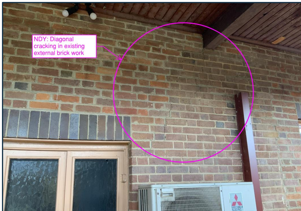
FIGURE 5 - VISIBLE DIAGONAL CRACKING IN AN EXTERNAL PERIMETER BRICK WALL
